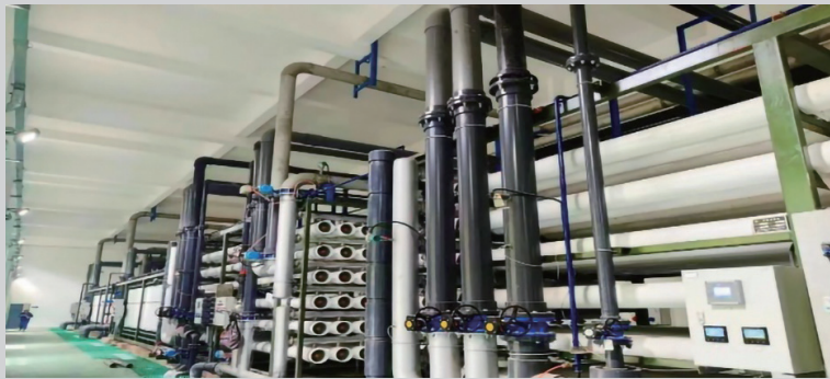
Special waste water treatment system
